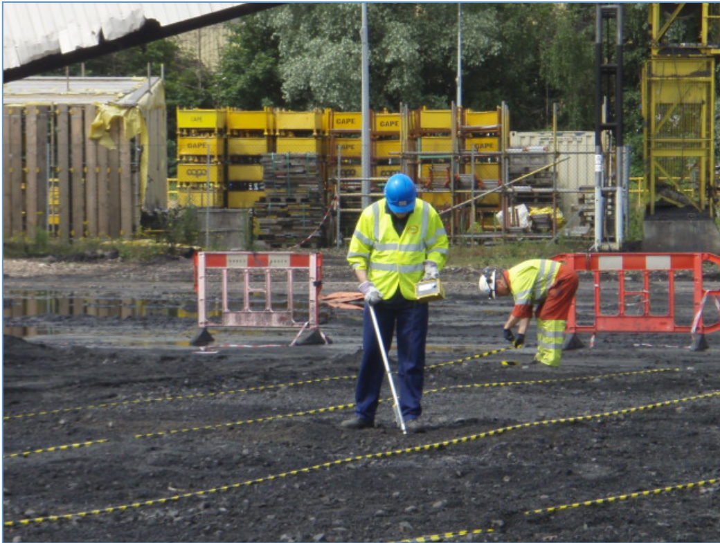
Picture of one of the radiological surveys undertaken to try to locate the missing source
